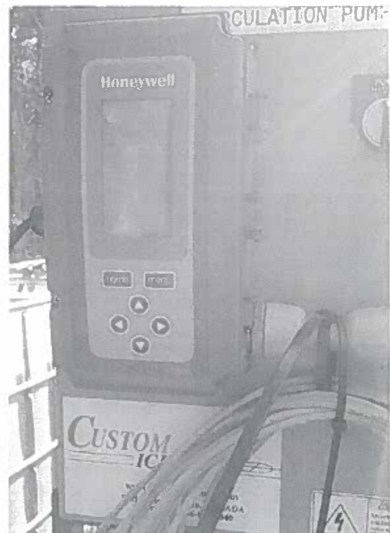
Circulation Pump Electrical Panel
