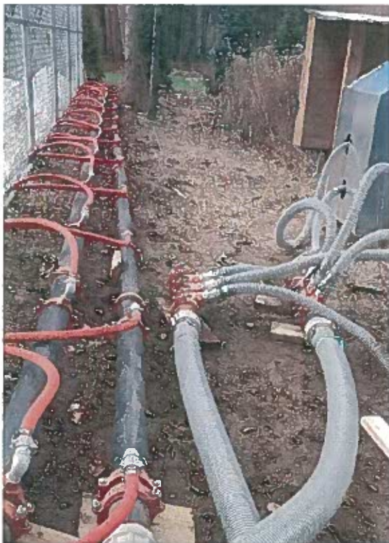
Cooling Supply Pipes
