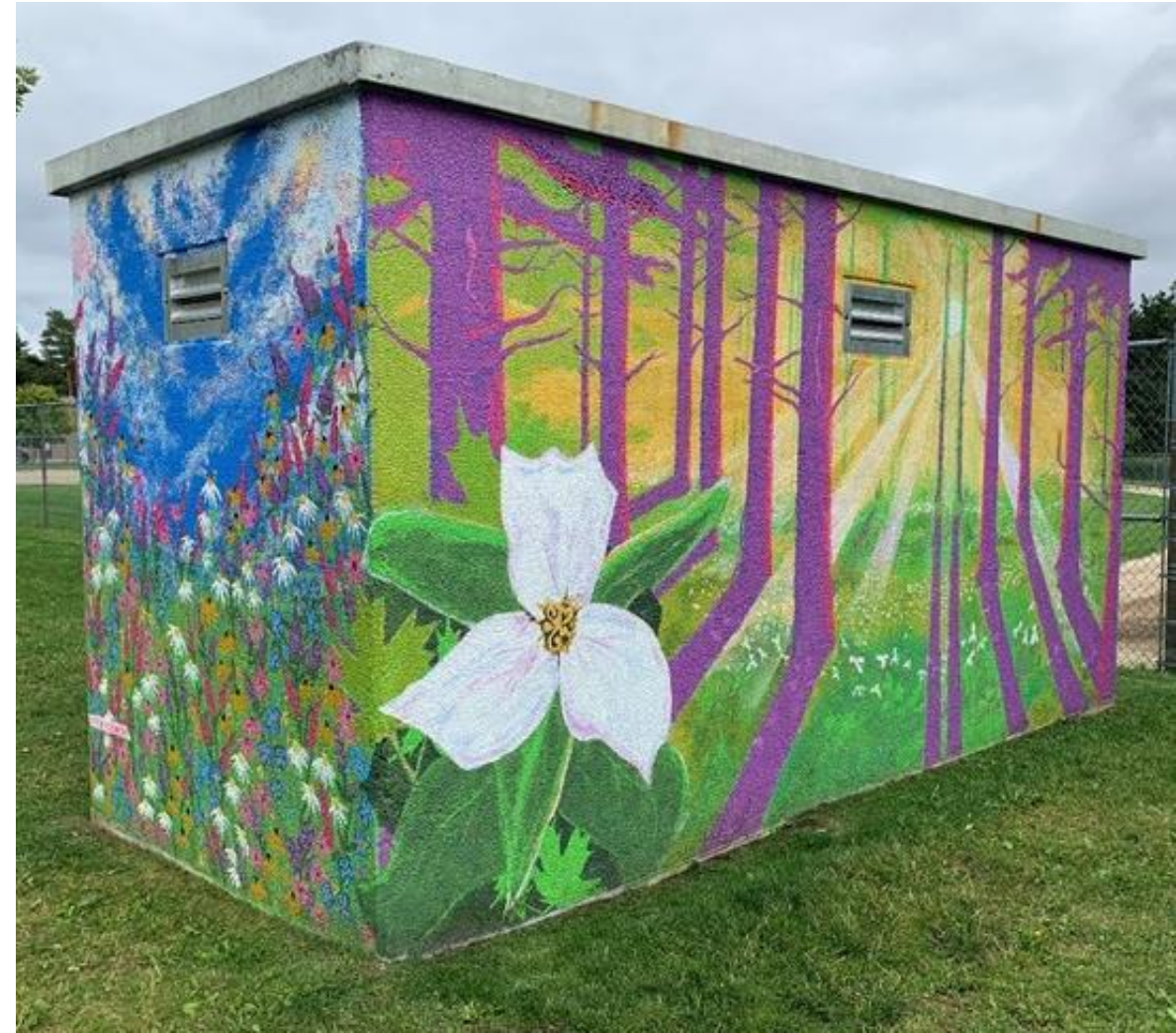
Lampman Lane Pumphouse Mural, by Scott Crew, Alexandra Gronfors, Monica Loney and Tiffany Symanski and under the mentorship of Katie Green, 2022
