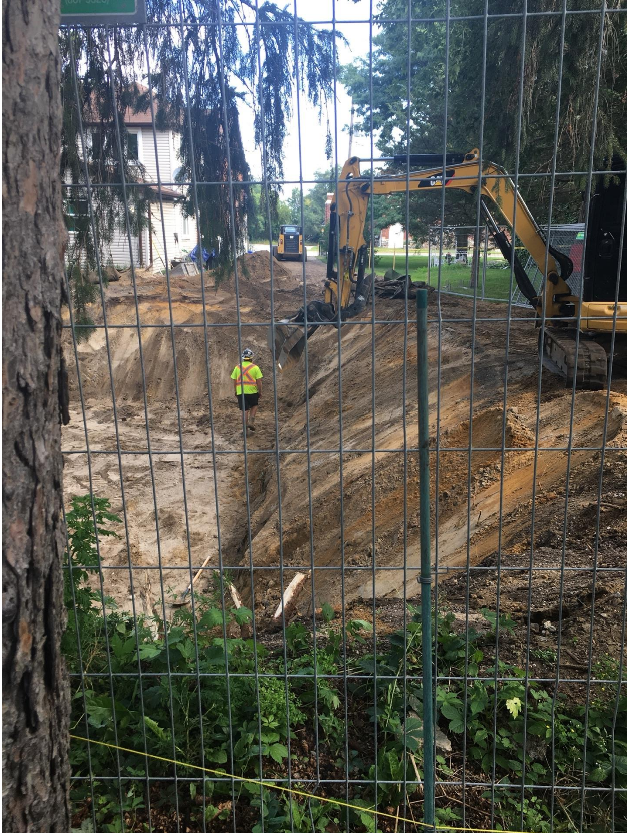
Aug 19, 2021: Unsafe pit excavation practices
