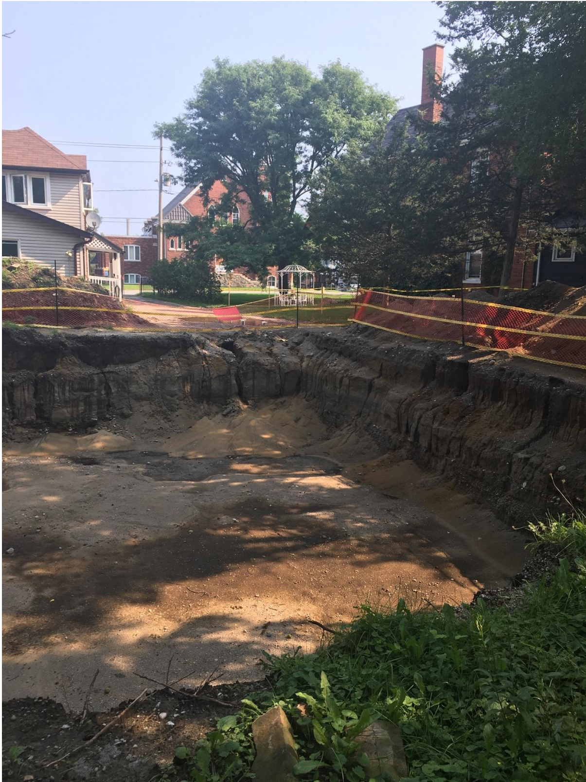
Aug 9, 2021: Pit sat idle for one month, unsafe erosion on vertical walls
