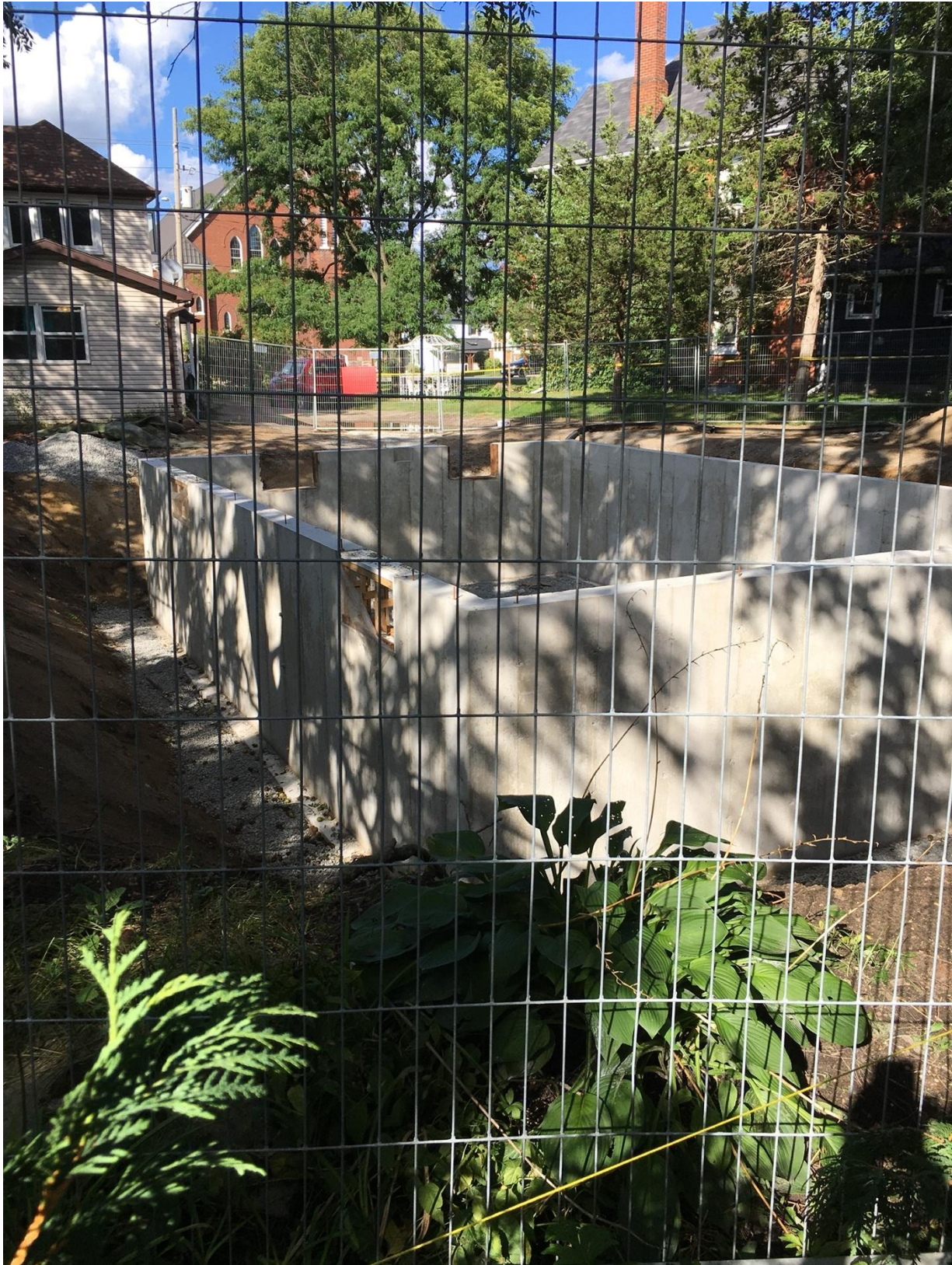
Sept 8, 2021: Site has sat idle for 3 weeks due to uneven walls
