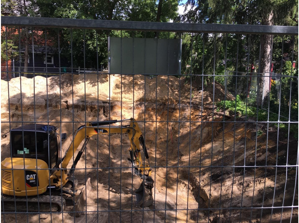
August 17, 2021: Further excavation means further damage to trees
