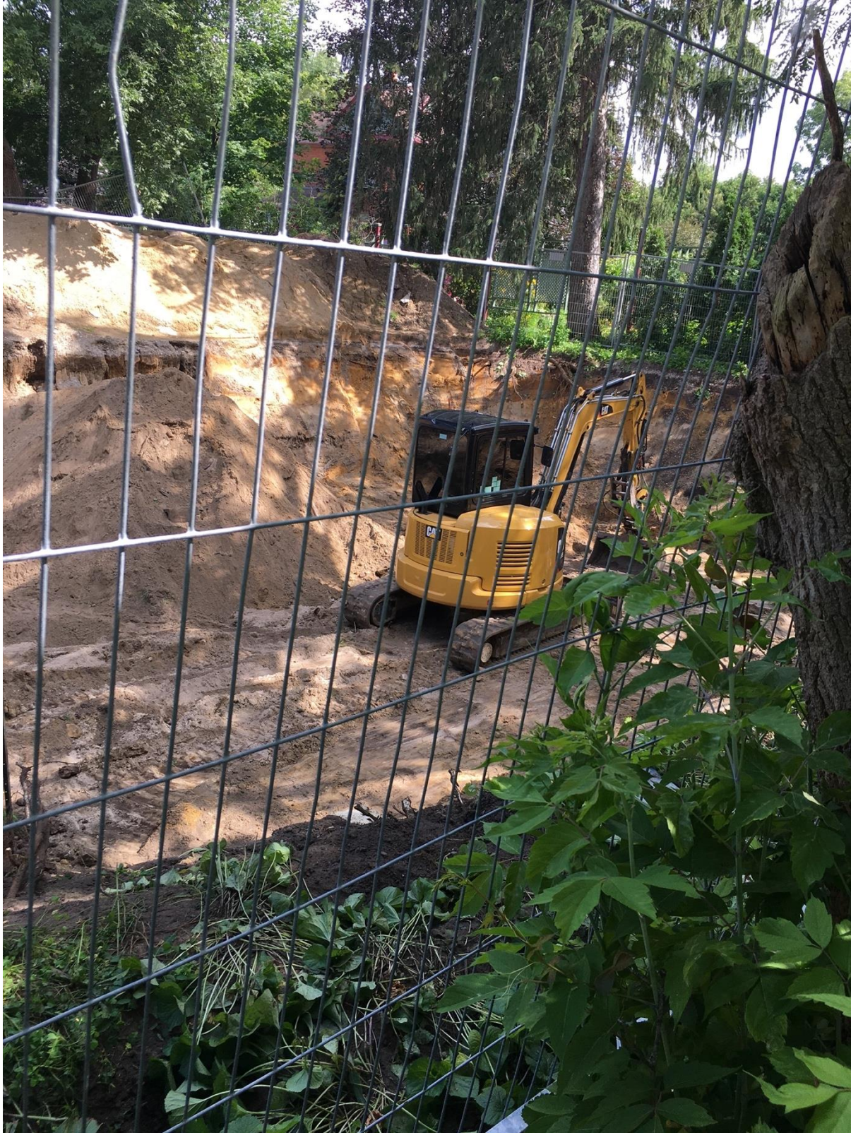
Aug 17, 2021: View showing pit encroaching on property boundaries damaging all boundary trees
