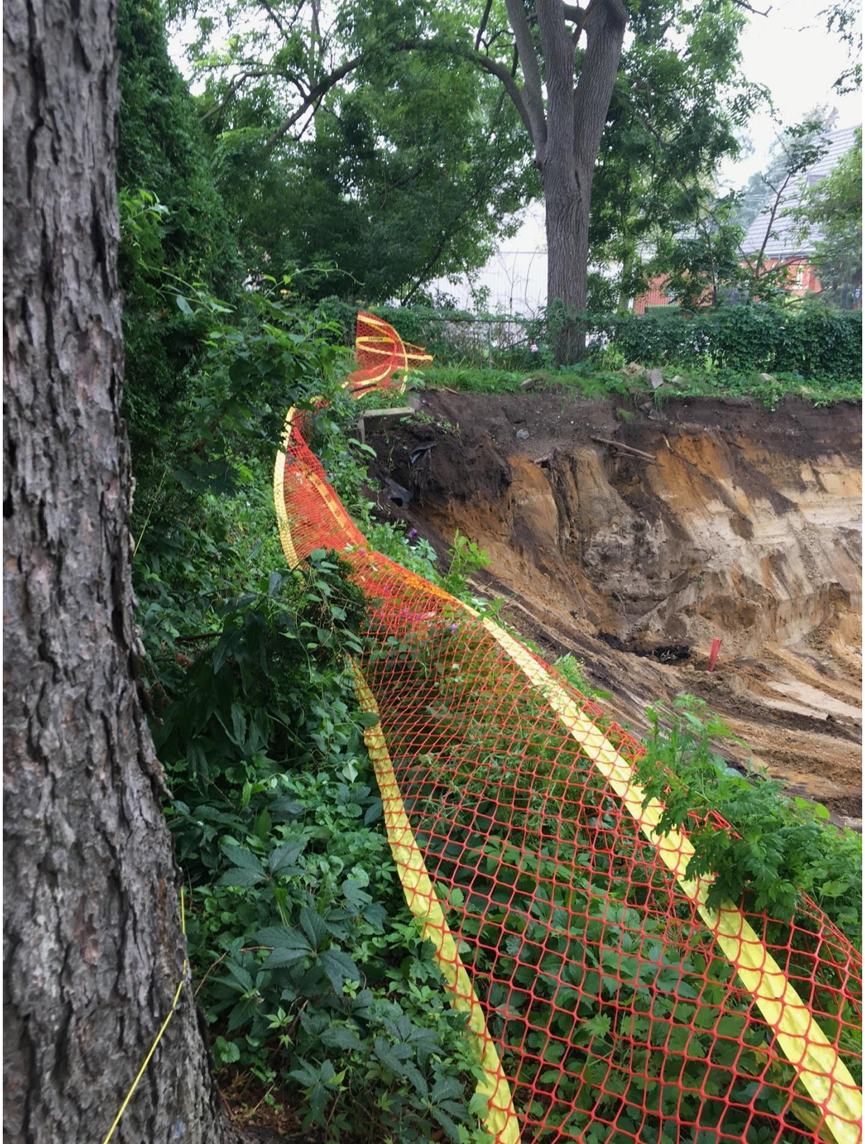
Aug 17, 2021: Further damage to Church's trees as slope is created to conform with Ministry's laws
