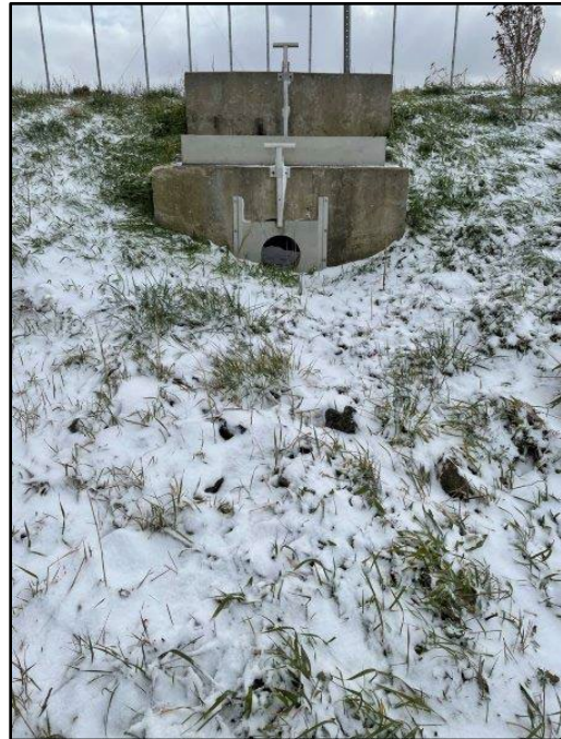
Image 62: Compost Pond Outlet Sluice Gate
