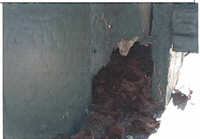
Photo #4: View of base of rotted post.
