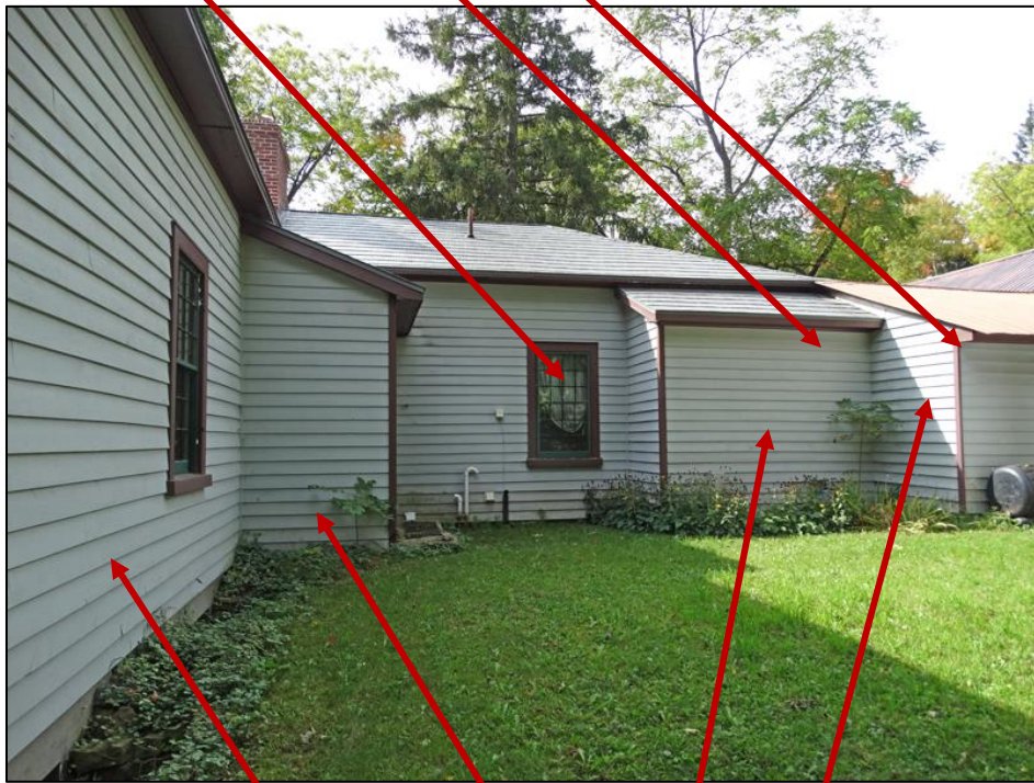
East façade showing L-R: house, 20 th century enclosure of centre hall doorway, original window, 20 th century enclosure of basement stairway, shed.
