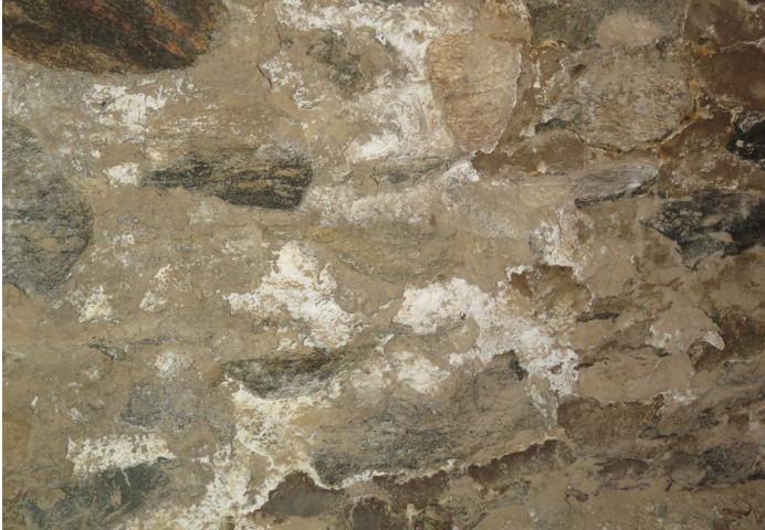
◀ Figure 4.9 Crawlspace efflorescence
