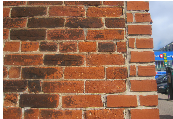
◀ Figure 4.12 Brick spall at south east corner where new and old brick meet
