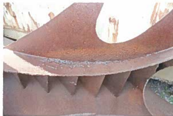
Filaments of steel from drilling of new drainage holes on the dragon's back
