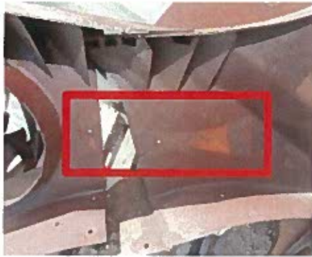
Bright orange corrosion product forming underneath connection joint
