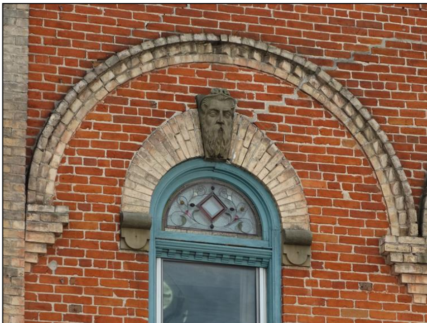
Figure 29: Window treatment showing the semicircular shaped opening, radiating brick voussoir (surround) with the portrait head keystone, terminating in terracotta stone (or stone) ends; with a tri-layer arch with corbelled plinth ends above, November 2021. The original window sashes have been replaced with a transom with art glass and a moulded frame. The lower sashes are modern.
