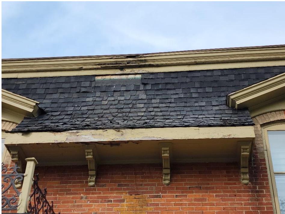
Image 1 – Photograph of area for repair of the mansard roof, and repair of the trim.
