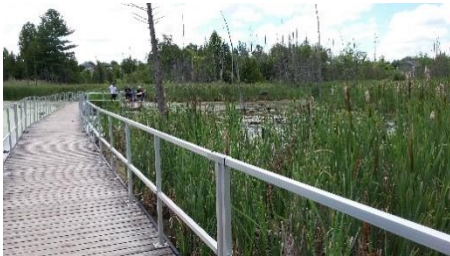
Bear Creek Eco-park Boardwalk requires board replacement, regular inspections and repair/re-installation of the railings.
